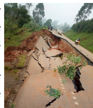
Roads washed away
